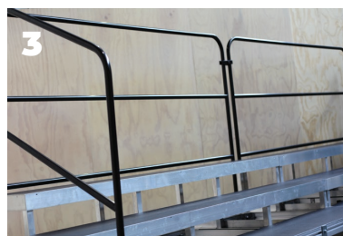
Your MELBA is now fully Installed.
